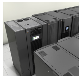
Liebert eXM adjacent to the wall
